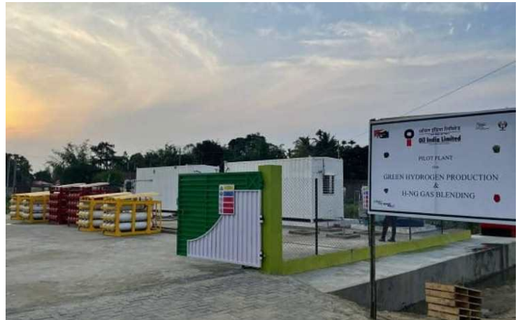
Figure 192: Green Hydrogen Pilot Plant at Oil India Limited's Jorhat Station (Source: T&D India)
