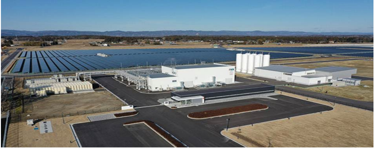
Figure 183: 10 MW alkaline water electrolysis system installed at Fukushima Hydrogen Energy Research Field (FH2R) (Source: FuelCellsWorks)
