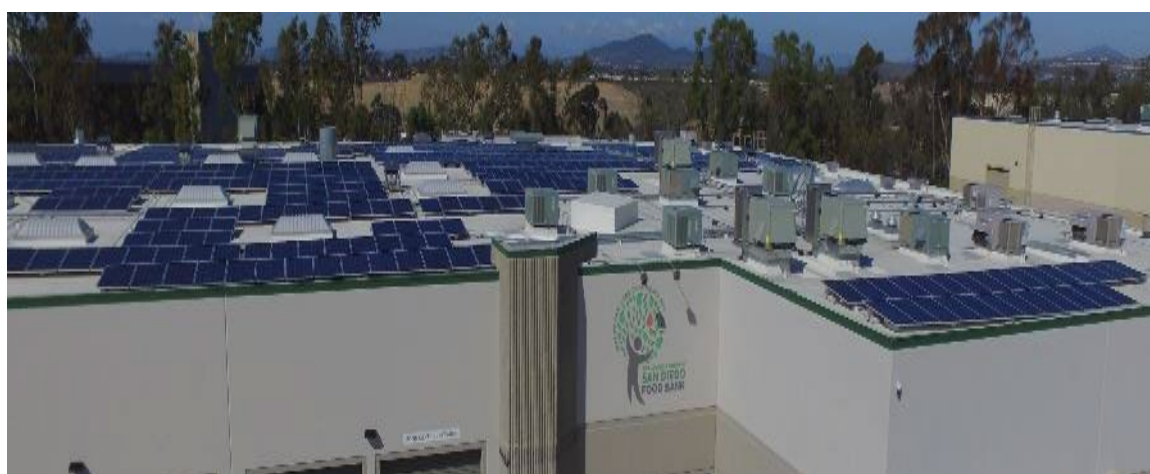
Figure 113: Solar panels installed at San Diego Food Bank 127
