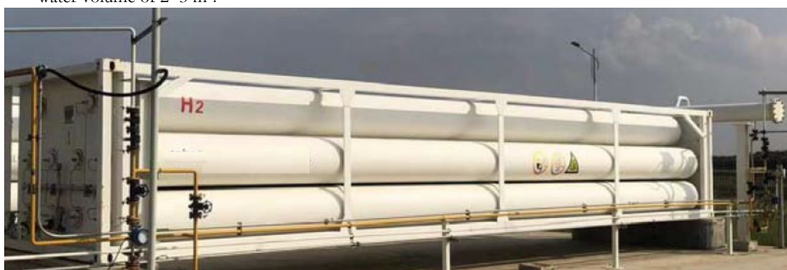
Figure 49: Hydrogen Tube Cascade/ Skid storage
