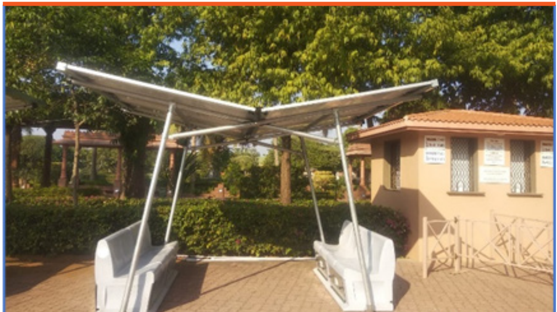
PV Port Systems installed in Swaminarayan Akshardham Mandir, Gandhinagar, Gujarat.
