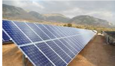
Solar PV power
